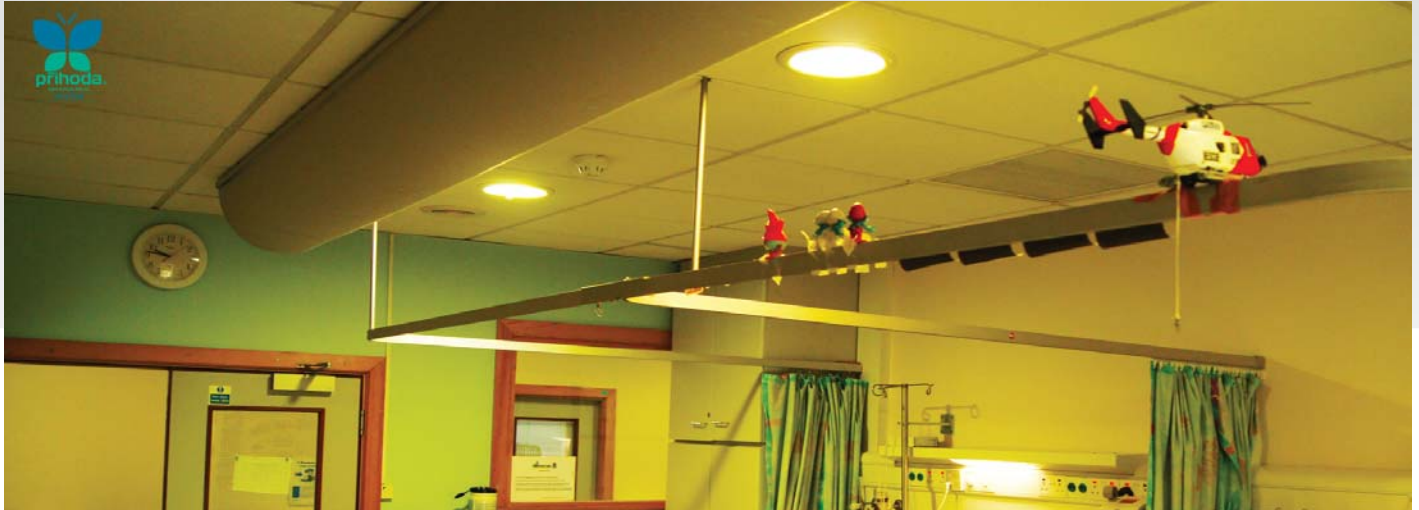
Light grey duct against light grey ceiling tiles.
