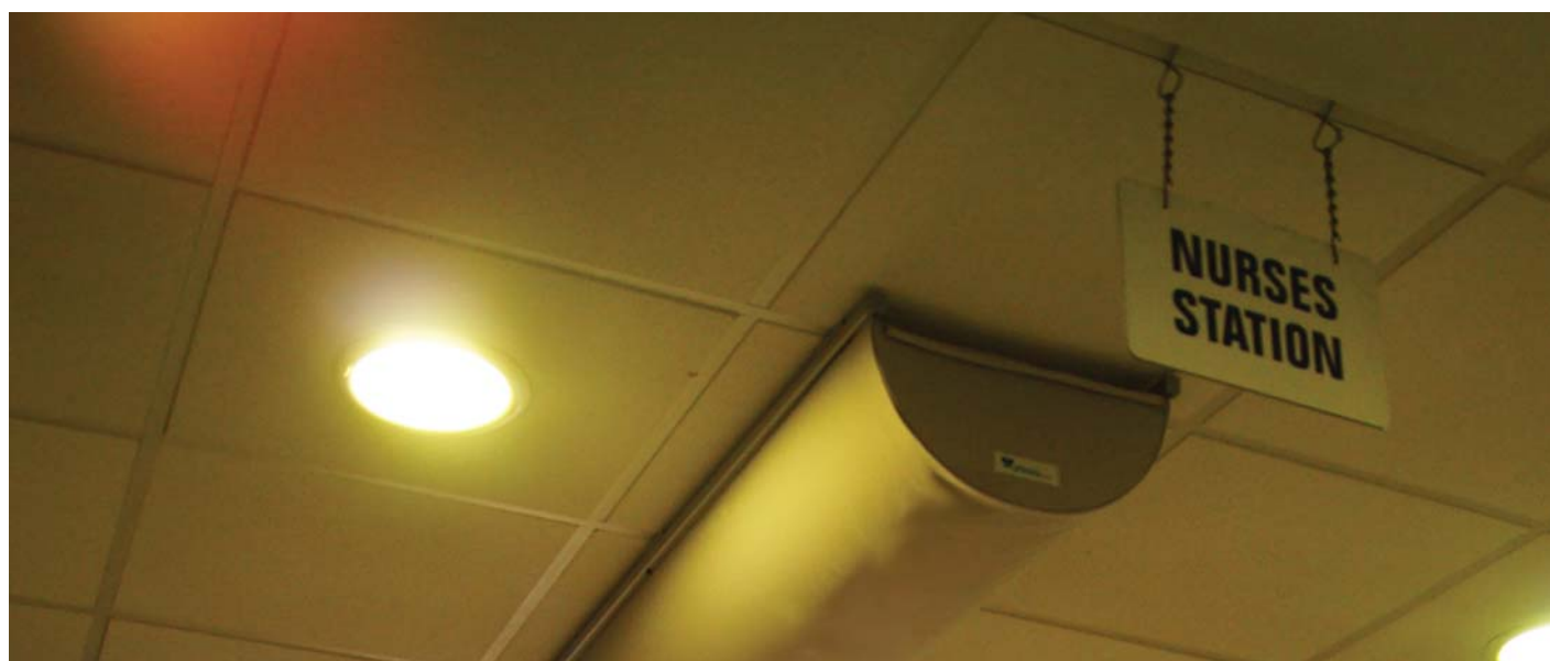
Cooling above the nurses station
