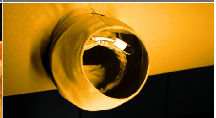
Damper for air volume correcting
