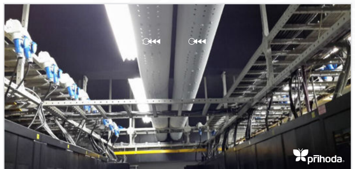
Server room, Leshan City, China
